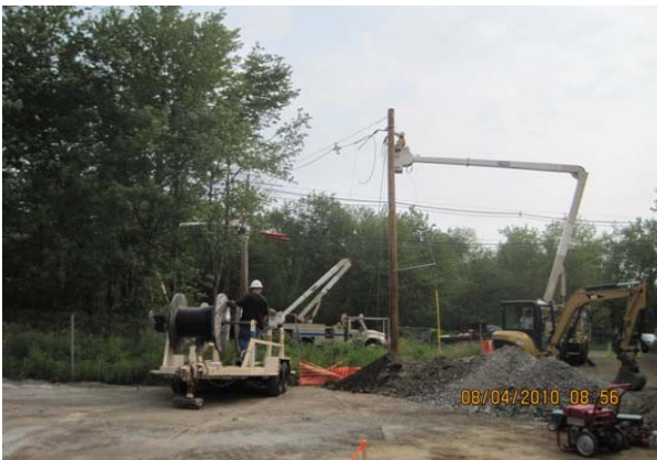
Middleton Electric tie in
