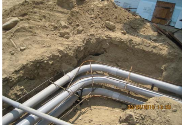
Electrical duct bank
